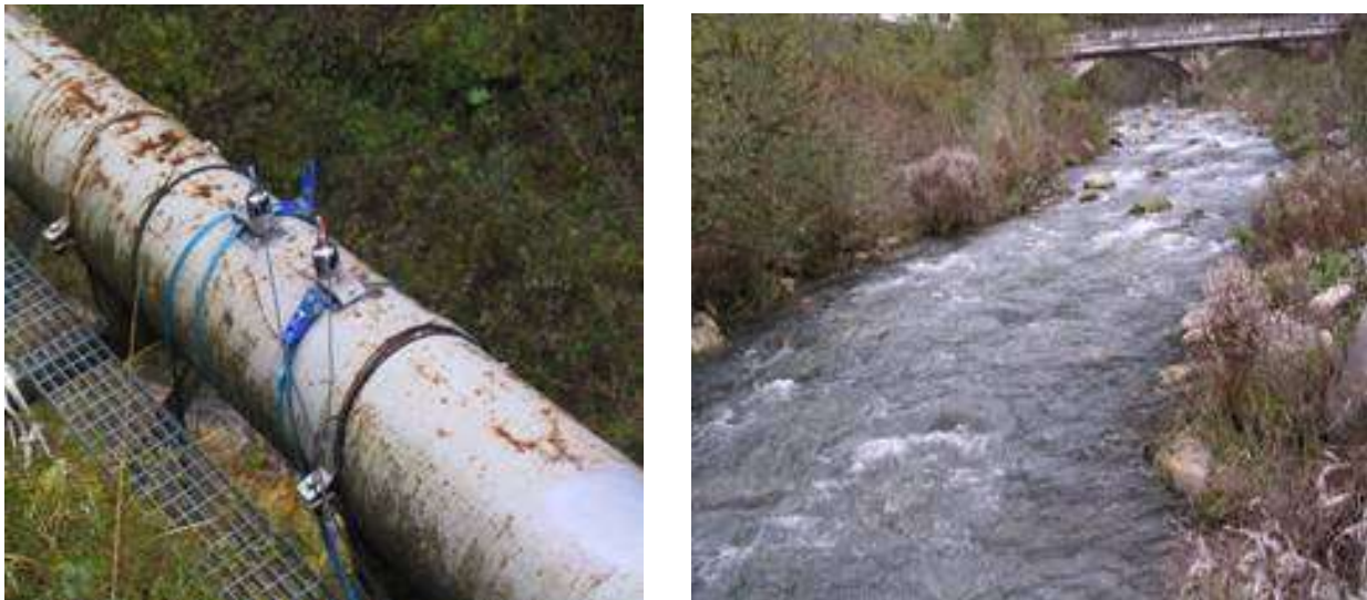
Figure 22: MIF measurements along the pipeline and just downstream Nervesa dam (Mis River)
