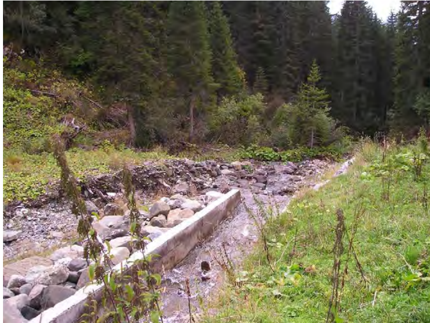
Figure 74: withdrawal point at 1639 m s.l.m.; small check dam and lateral channel for DMV ensurance
