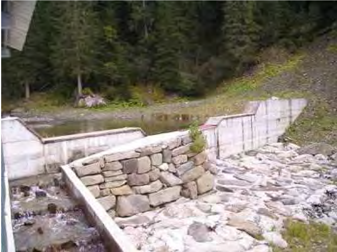
Figure 61: Hydropower plant on which the MCA method will be applied.
